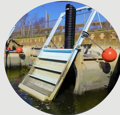
SELF REGULATING TIDE GATE INSTALLED ON BAY SIDE OF CULVERT
